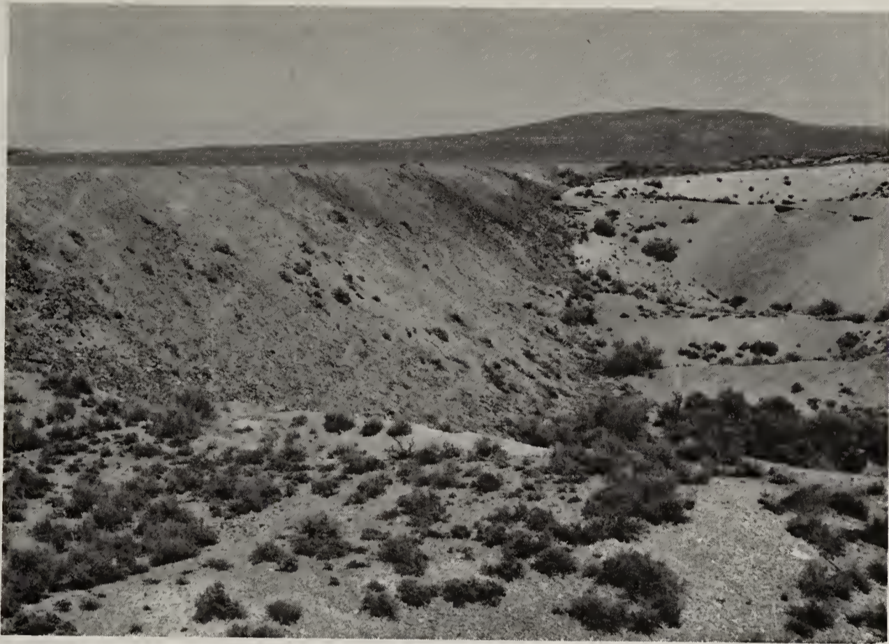
Figure 91: The large earthen fill carries the railroad over Dove Creek Sink. (BLM photo)
